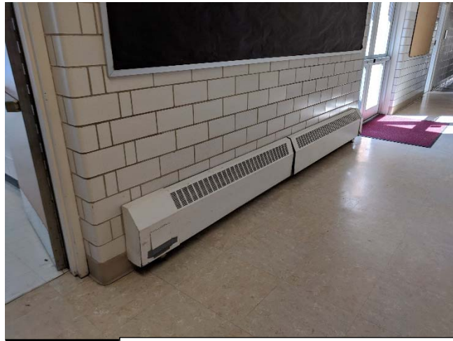
Photo #18 Typical Fin Tube Radiator
