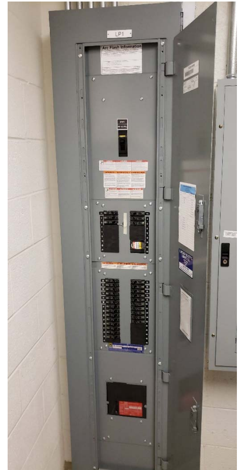
Photo #12 Typical Branch Panelboard installed in 2015
