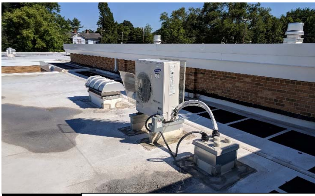
Photo #20 Typical Split DX Condenser Unit
