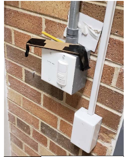
Photo #20 Typical Wall Mounted Occupancy
