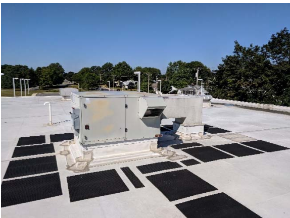
Photo #9 Typical Energy Recovery Unit
