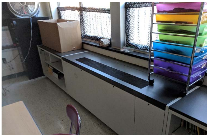
Photo #10 Typical Unit Ventilator
