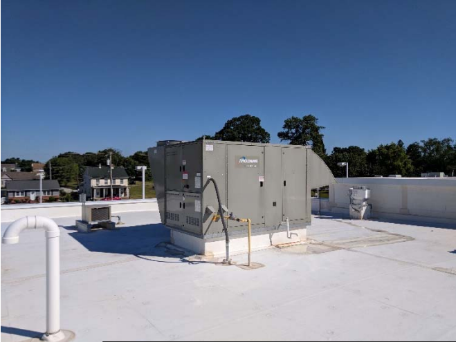
Photo #11 Packaged DX Rooftop Air Handling Unit serving Kitchen
