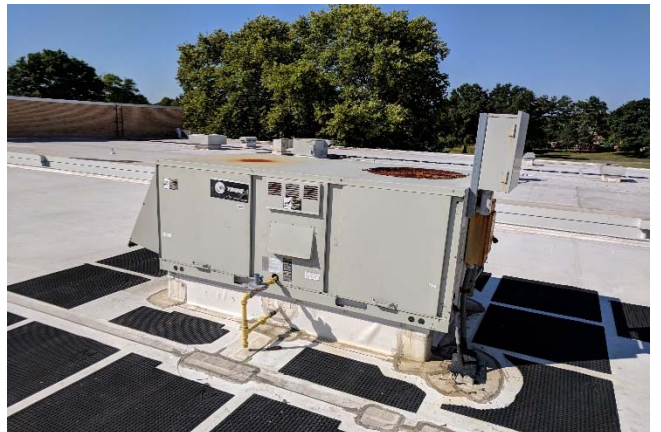
Photo #8 RTU Serving Library
