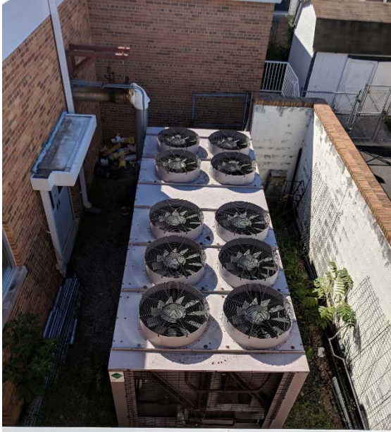
Photo #1 Air Cooled Chiller
