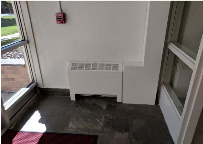
Photo #23 Typical Vestibule Cabinet Heater
