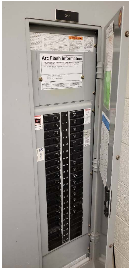
Photo #11 Typical Branch Panelboard installed in 2002
