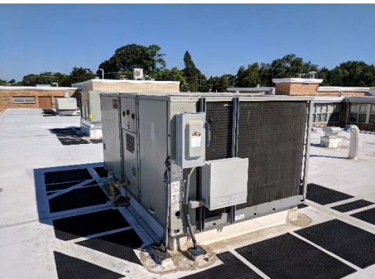
Photo #19 Typical Packaged DX Rooftop Air Handling Unit
