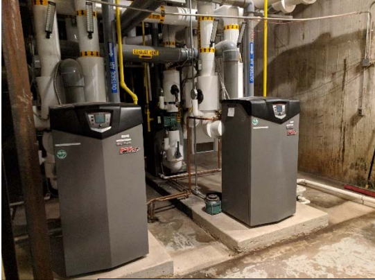
Photo #15 Typical Boilers in Mechanical Room
