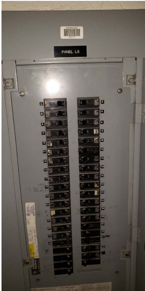
Photo #10 Typical Branch Panelboard installed in 1993
