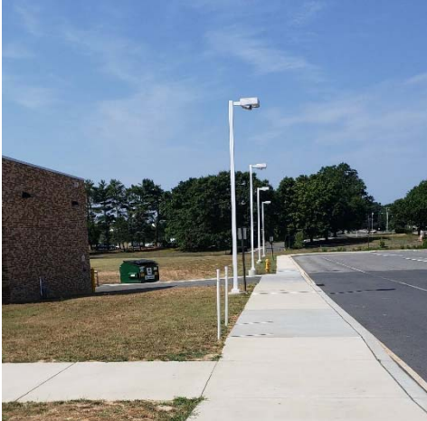
Photo #16 Typical LED Parking Lot Lights
