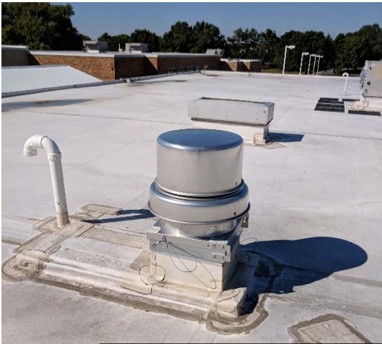
Photo #17 Typical Exhaust Fan
