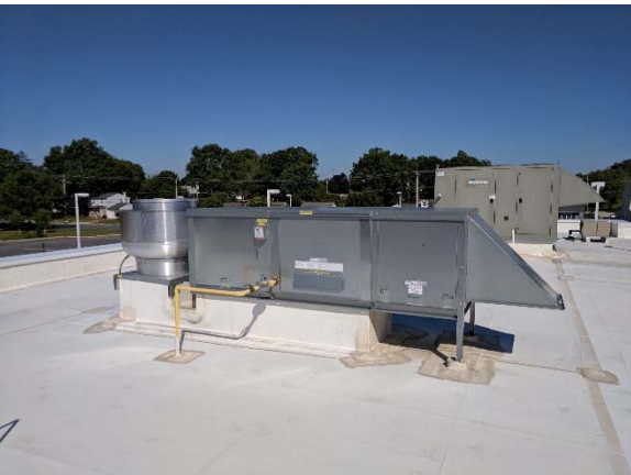
Photo #7 Kitchen Makeup Air and Exhaust Unit
