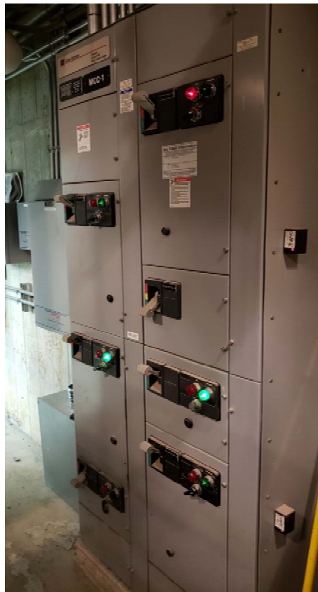
Photo #3 Motor Control Center
