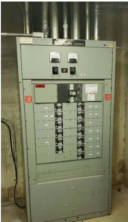
Photo #7 Switchboard MDP
