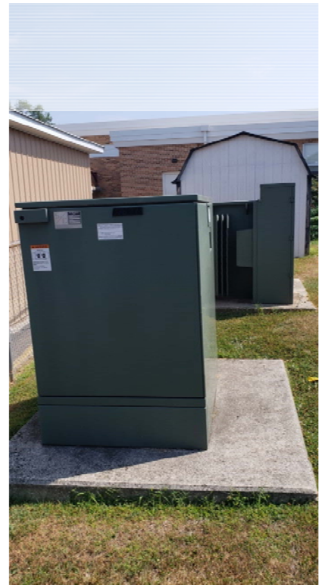
Photo #4 PMH-3 Switch and 500kVA Transformer
