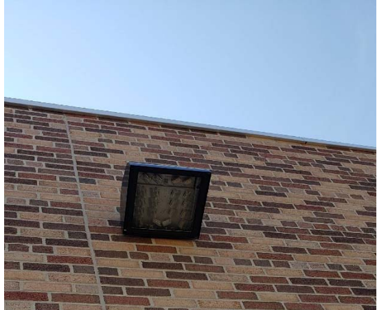
Photo #17 Typical LED Wall Mounted Light on Kitchen Exterior Walls
