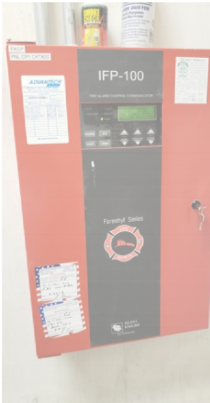
Photo #2 Fire Alarm Control Panel
