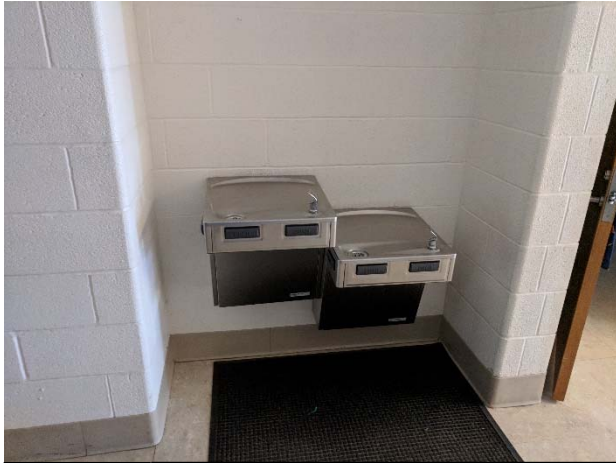
Photo #21 Typical Water Fountain
