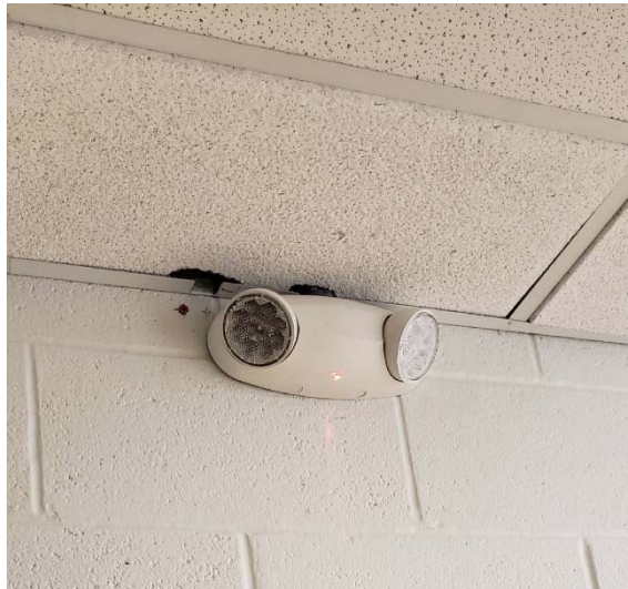
Photo #19 Typical Wall Mounted Emergency Light
