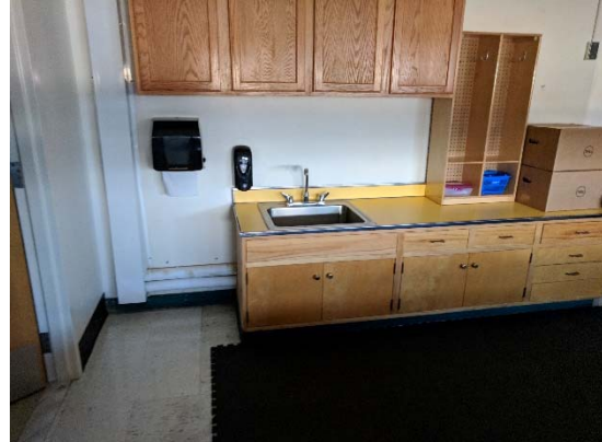
Photo #16 Typical Classroom Sink
