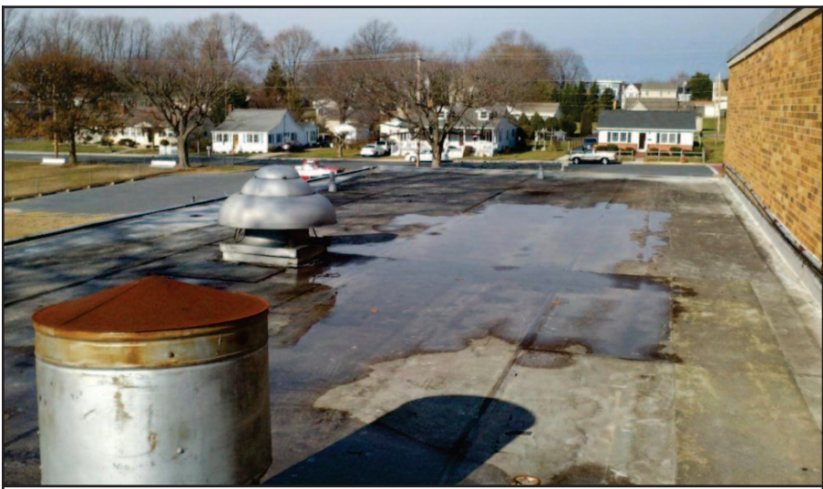
SES Roof - ponding & blistering due to exceeding lifespan
