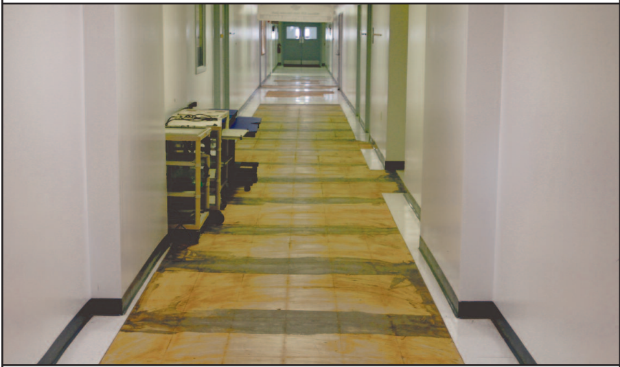
Thomas D. Clayton Building, that houses the SSD Technology Center, has many structural and HVAC issues
