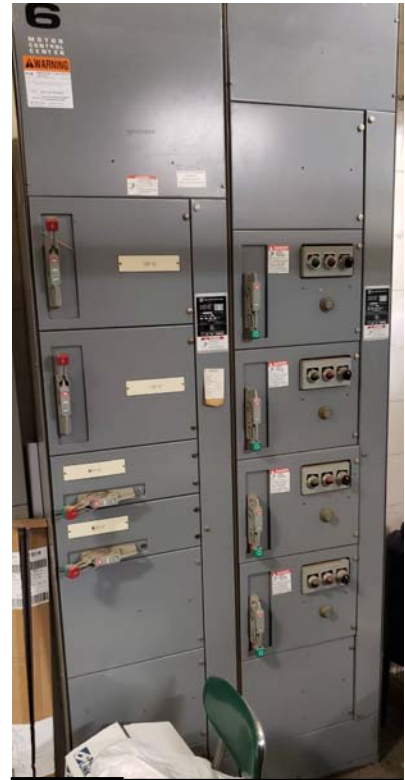
Photo #3 Motor Control Center
