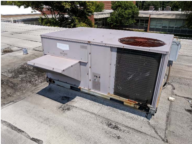
Photo #11 RTU serving Library
