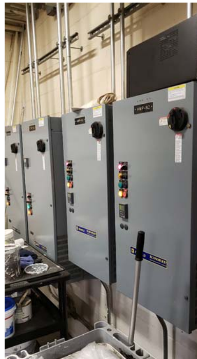
Photo #20 Typical VFD
