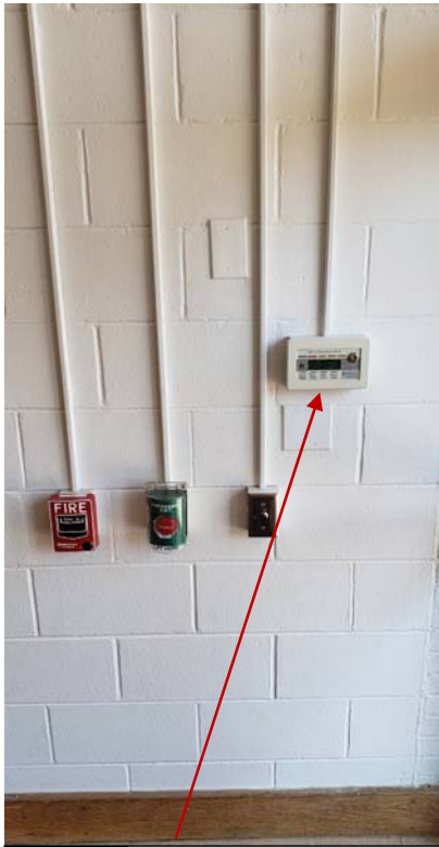
Photo #1 Fire Alarm Annunciator Panel
