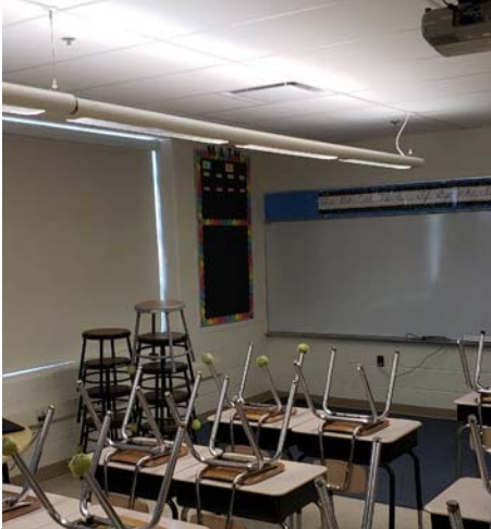
Photo #11 Typical 2006 Addition Classroom Lighting
