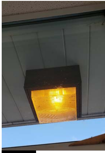
Photo #17 Typical Light under Canopy
