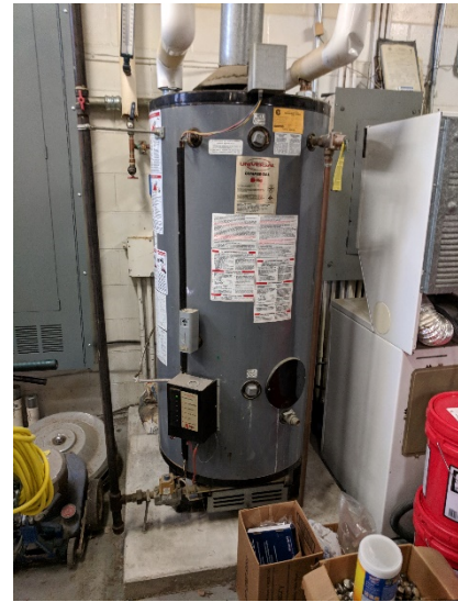
Photograph #6 – Domestic Water Heater
