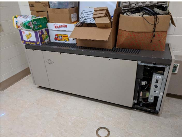
Photo #16 Typical Unit Ventilator
