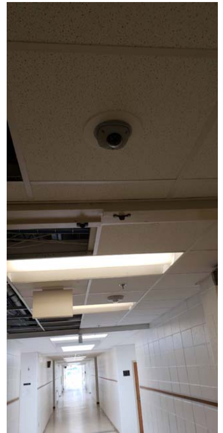
Photo #15 Typical Interior Video Surveillance
