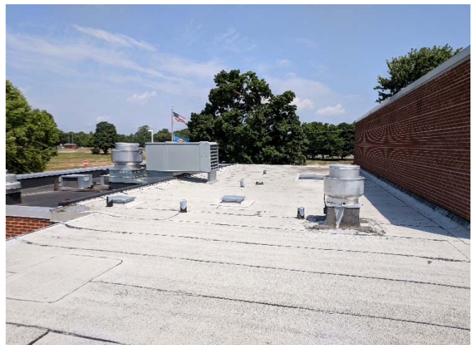
Photo #6 Kitchen Mechanical Equipment on Roof
