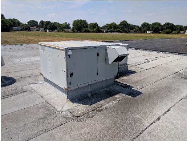
Photo #12 Typical Energy Recovery Unit
