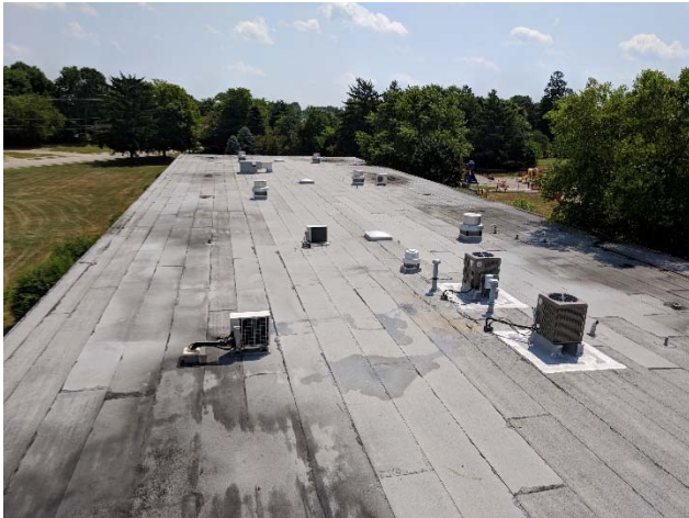
Photo #3 D Wing Roof Mechanical Equipment
