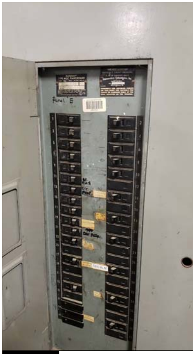
Photo #4 Panelboard E is past useful service life
