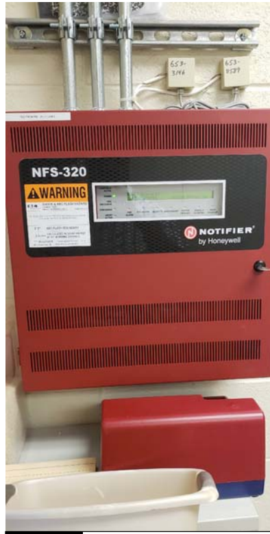
Photo #2 Fire Alarm Control Panel
