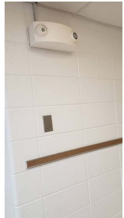
Photo #21 Typical Wall Mounted Emergency Light Fixture
