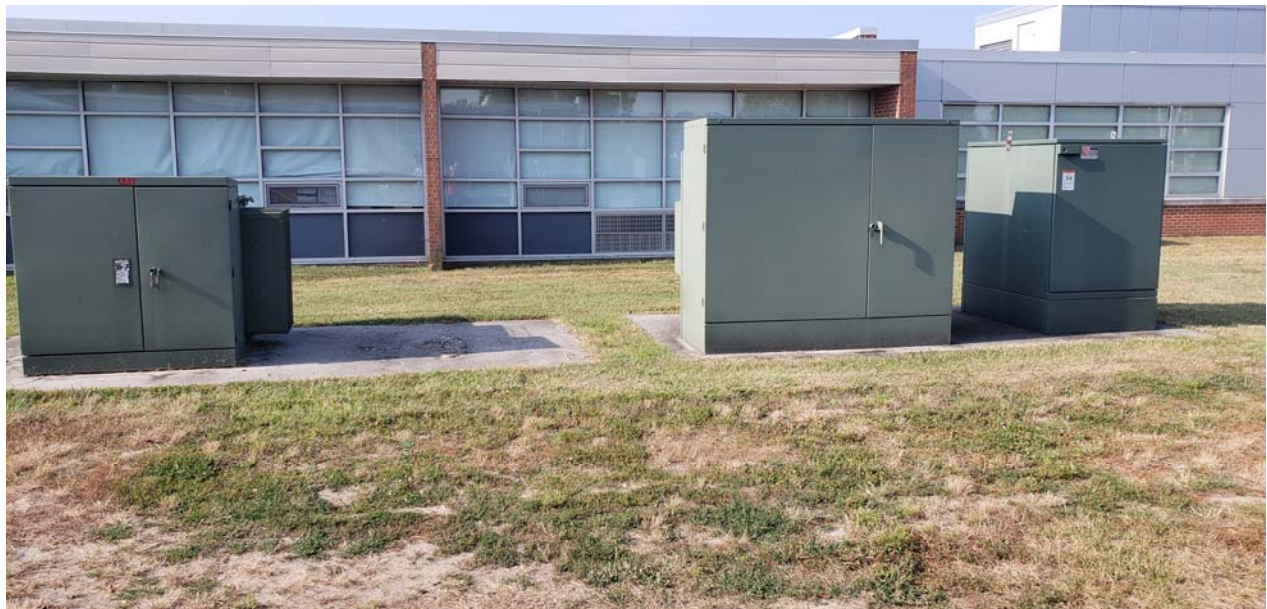
Photo #10 Transformer and PMH-3 Switch
