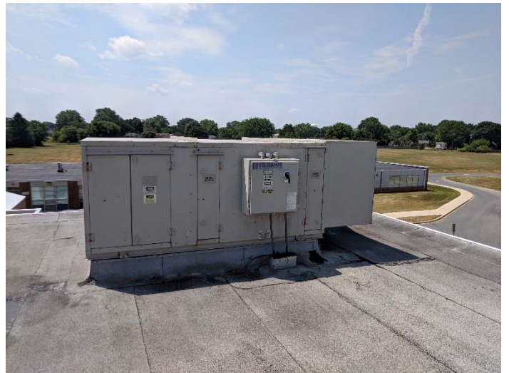
Photo #10 Gym RTU
