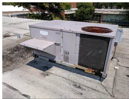
Photograph #4 – RTU Serving Library
