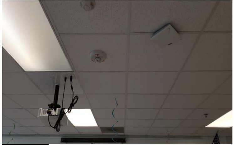
Photo #12 Typical Classroom with Occupancy Sensor
