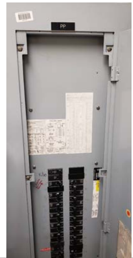
Photo #18 Typical Panelboard installed in 1993
