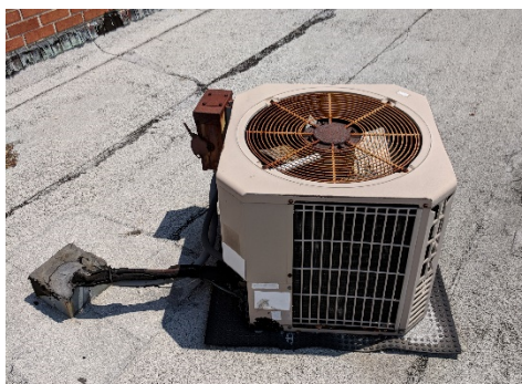
Photograph #3 – DX Split System Condensing Unit
