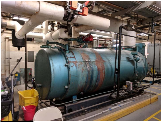
Photo #9 Backup Boiler in Mechanical Room
