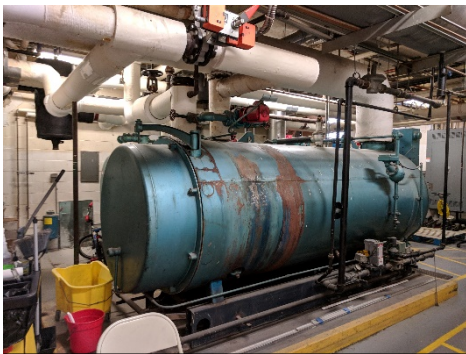
Photograph #1 – Backup Boiler in Mechanical Room
