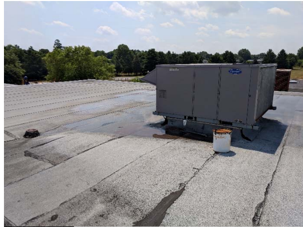
Photo #13 Cafeteria RTU
