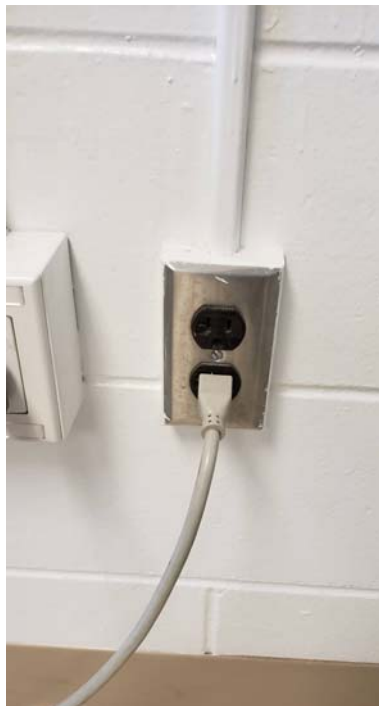
Photo #19 Typical Surface Mounted Receptacle
