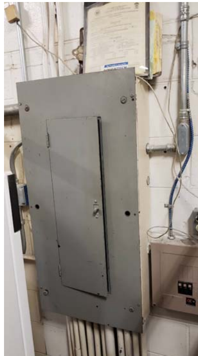
Photo #5 Panelboard E
