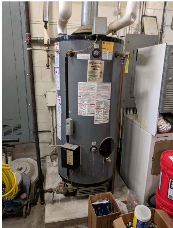
Photo #15 Domestic Water Heater
