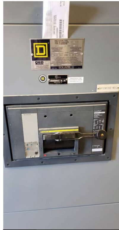
Photo #9 Switchboard MDS2
