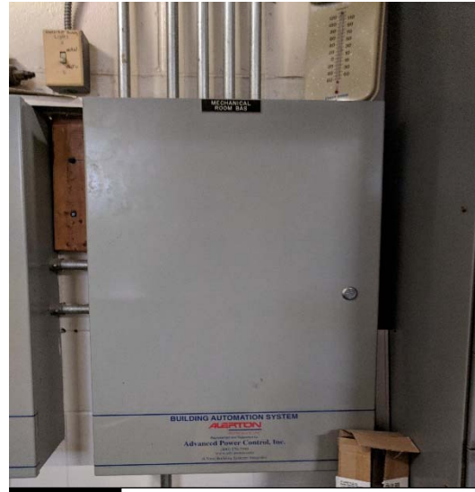
Photo #2 BAS Control Panel
