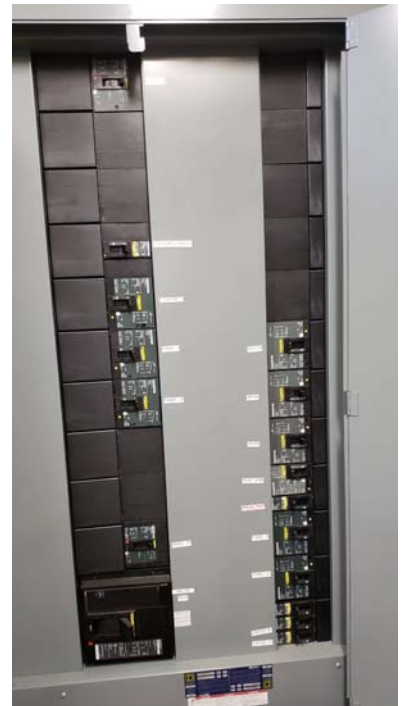
Photo #6 Panelboard MDP
