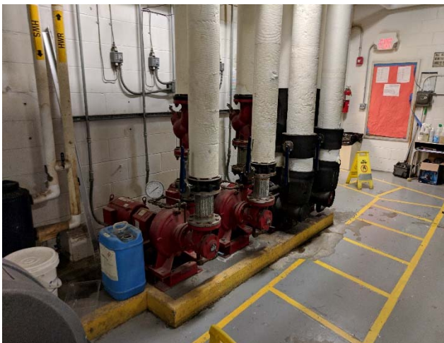
Photo #5 Hot and Chilled Water Pumps in Mechanical Room
