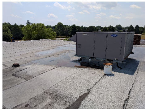
Photograph #2 – Cafeteria RTU
