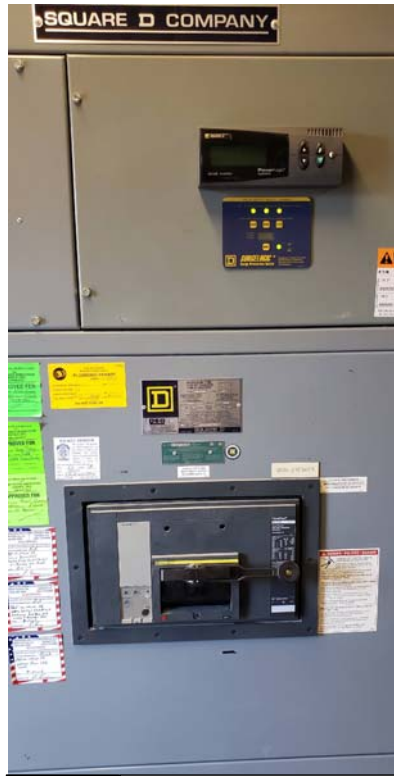
Photo #8 Switchboard MDS1
