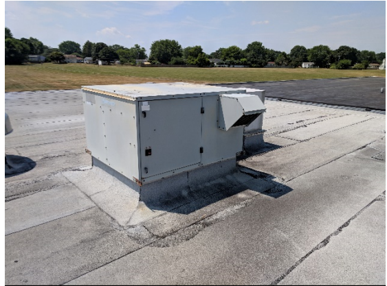
Photograph #5 – Typical Energy Recovery Unit
