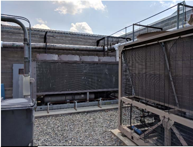
Photo #1 Air Cooled Chillers
