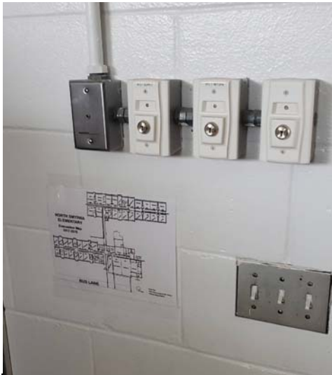
Photo #16 Typical Light Switches and Remote Test Switches
